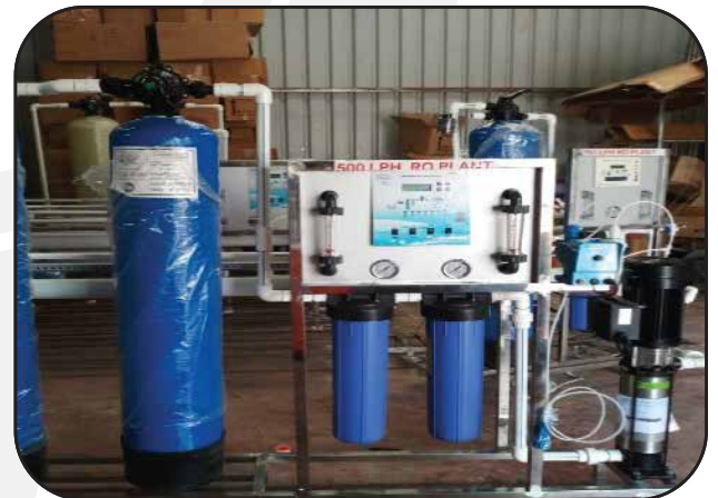
RO PLANT WITH WATER ATM
